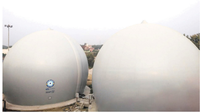
140 MLD STP at Dinapur, Uttar Pradesh
